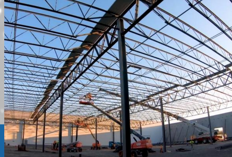
Expansion & construction of magnesium module 1B at our JV plant GF Linamar, USA
